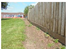
This path leading to the gardening area is also being resurfaced and
